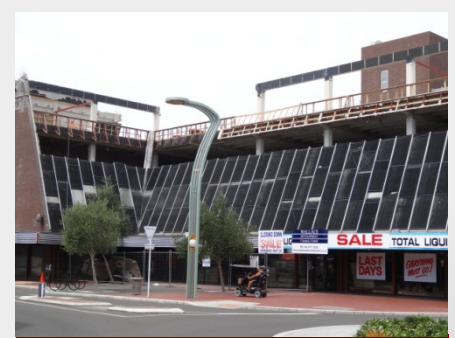
Wallace Development progress the redevelopment of the former Power Board building due for completion in May. Hawke's Bay Today will occupy the first floor.
